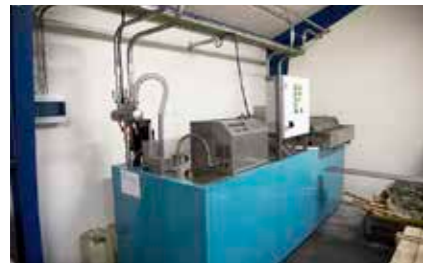
The central filtration system for filtering coolant.
