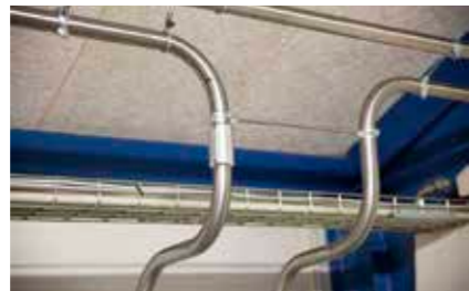
We provide you with a turnkey solution including installation work such as piping.
