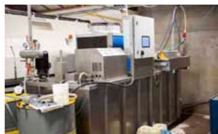
The central filtration system for filtering coolant.
